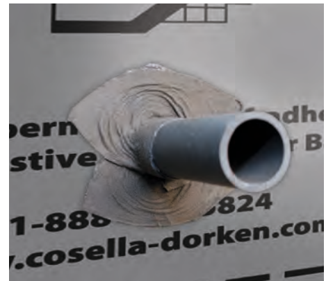
Air barrier continuity at penetrations
